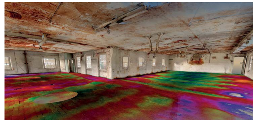
BOAR'S HEAD MILLS, DARLEY ABBEY: LASER SCAN OF LONG MILL, SHOWING LOWER FLOOR AREAS (RED AND PURPLE) WORN BY WORKERS AS THEY MOVED AROUND THE MACHINES, ADDING TO UNDERSTANDING OF THE INTERNAL ORGANISATION OF THIS BUILDING. THIS PROJECT WAS CARRIED OUT AS PART OF THE HERITAGE LOTTERY FUNDED YOUNG ROOTS PROJECT. SOURCE: DERBYSHIRE COUNTY COUNCIL.
